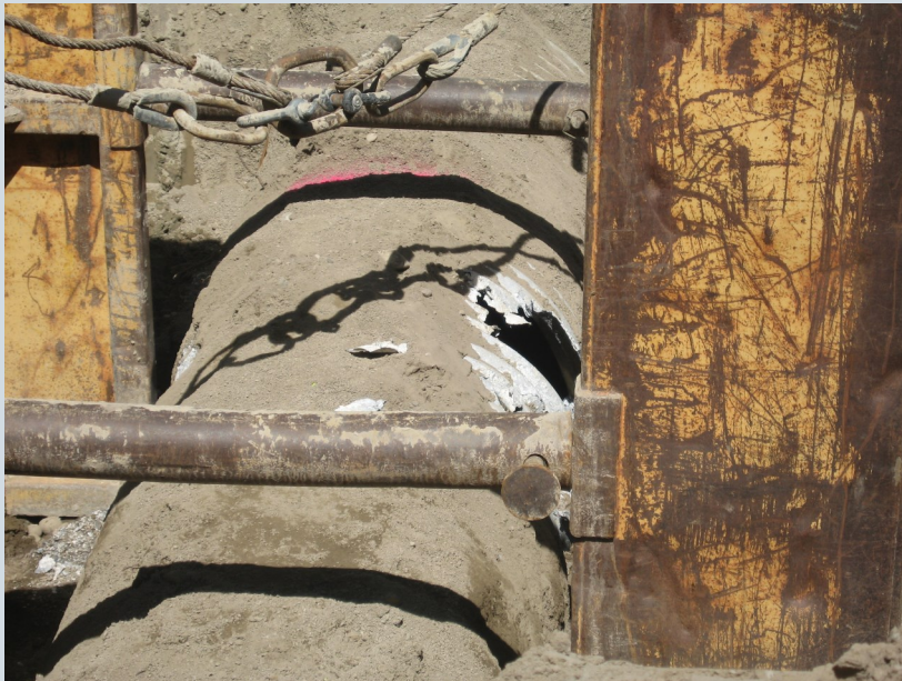
Picture shows deterioration of outfall pipe
