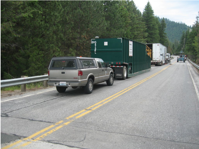
Collection Tank (aka Baker Tank) Used to collect debris and water
