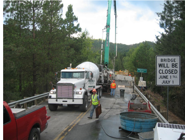
Concrete Truck and Pump set up at the end of the bridge
