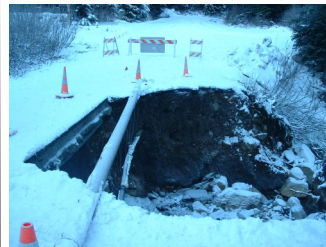
(Left) Wash out of culverts .
