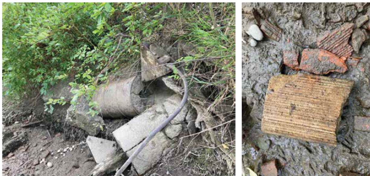
FIGURE 15. DEBRIS IN THE RIVER BANK NEAR SITE 13
