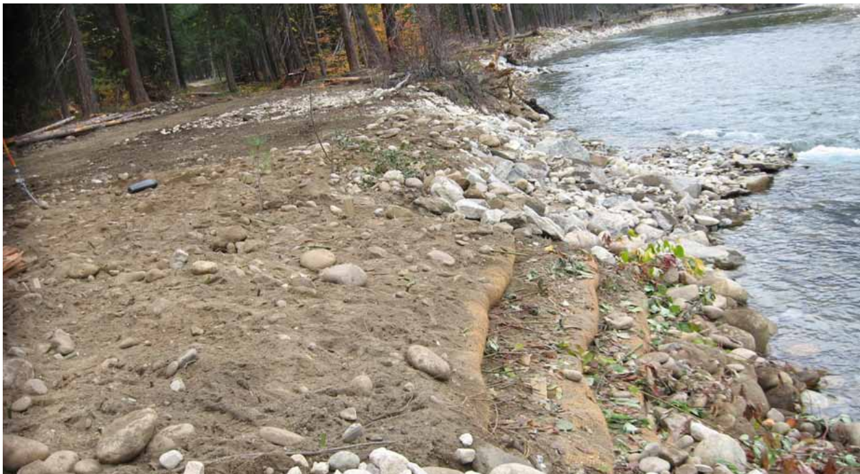
Photo 11 – Rock barb and willow layers (bioengineering) on upper Company Creek Road shortly after installation.
