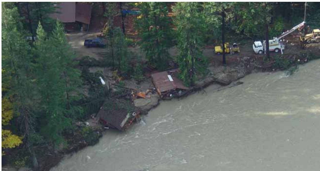
Photo 31 – Destruction of private cabin and damage to upper Company Creek Road during the 2003 flood.
