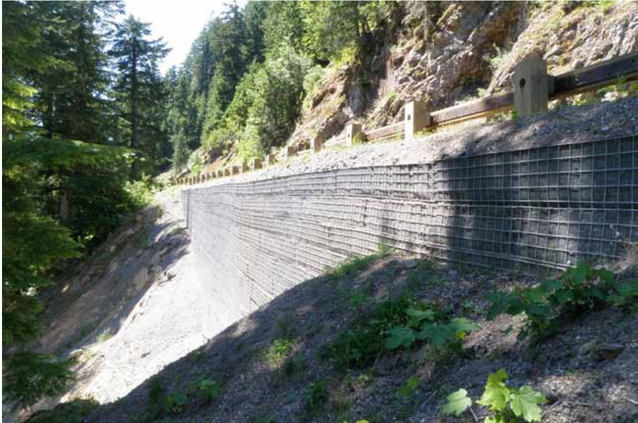
Figure II-7: An example of a Mechanically Stabilized Earth (MSE) Wall from Mount Rainier National Park (similar to the wall that is proposed in Alternative 5)
