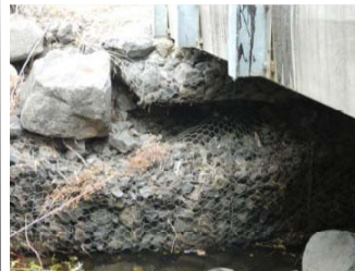
(Left) Failing Gabion on Stone Hill Bridge #915
