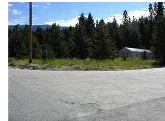
(Left) Condition of Chiwawa Loop Road.
