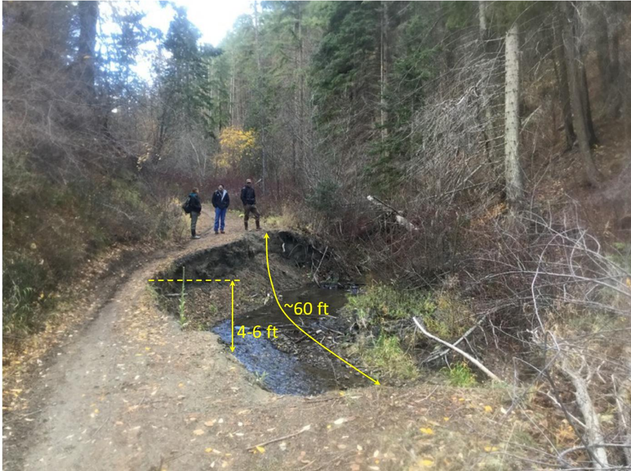
Approximate dimensions of road washout, looking upstream at washout area.
