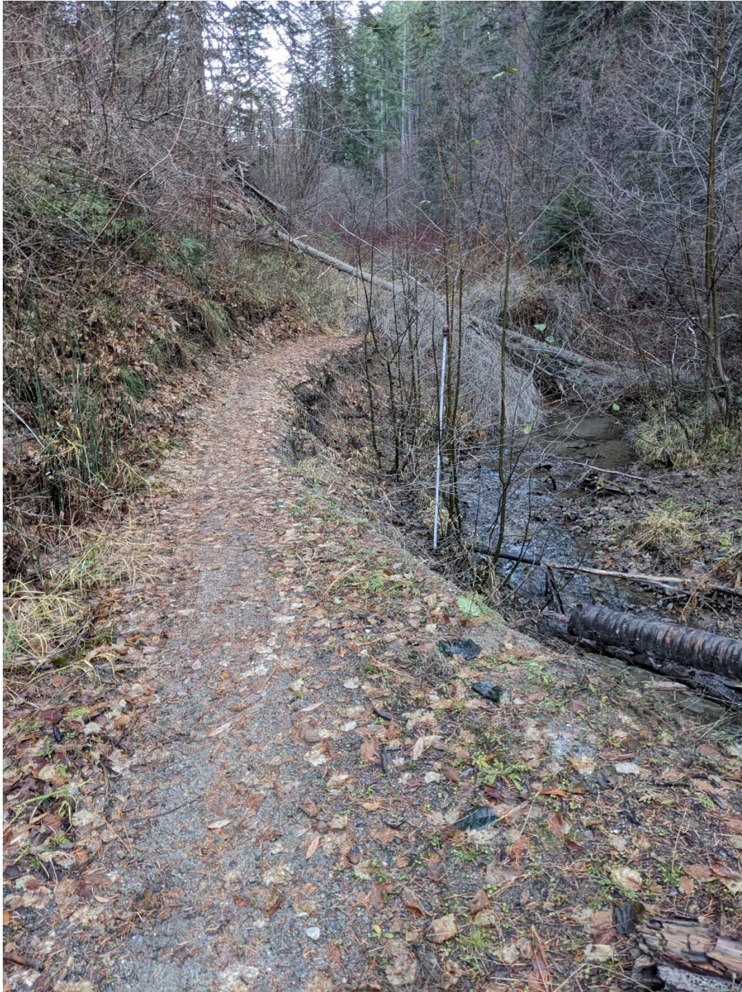
Road washout approximately halfway through project area. Not associated with floodplain grading or logjam placement.
