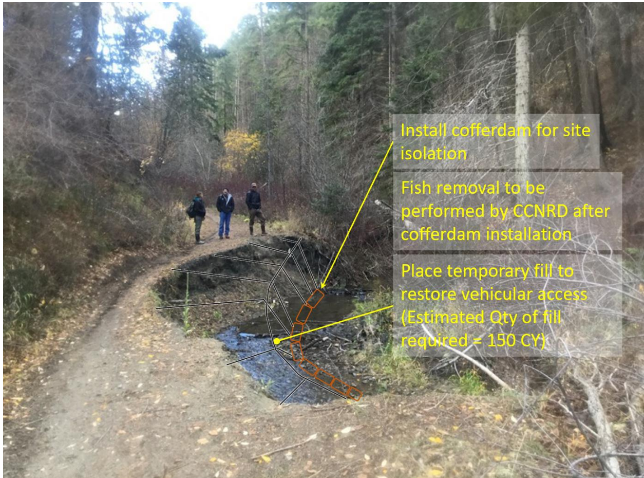
Site isolation needs for road washout.
