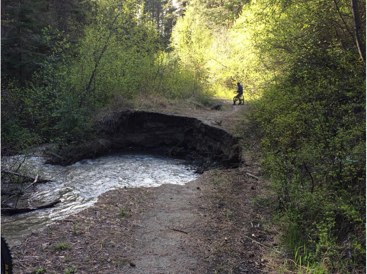
Looking downstream at washout area.
